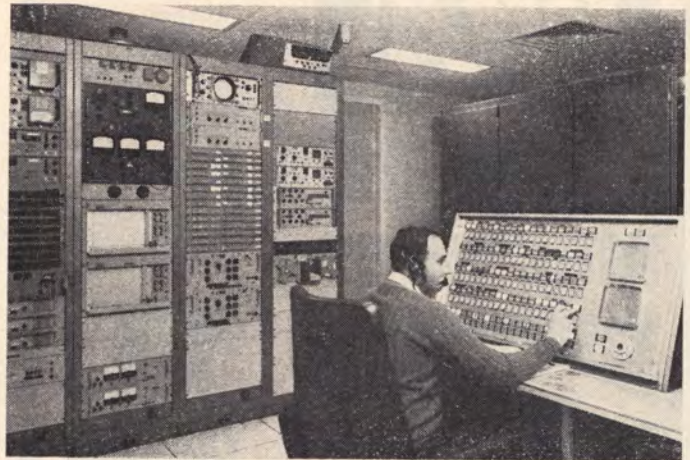
NASA Switching Center at Deakin (Canberra): Voice communications switching board, linking all Australian tracking stations with the world-wide NASA communications network. The same circuits are used for conversations between the astronauts and the Apollo Mission Control Center at Houston, Texas, U.S.A.
