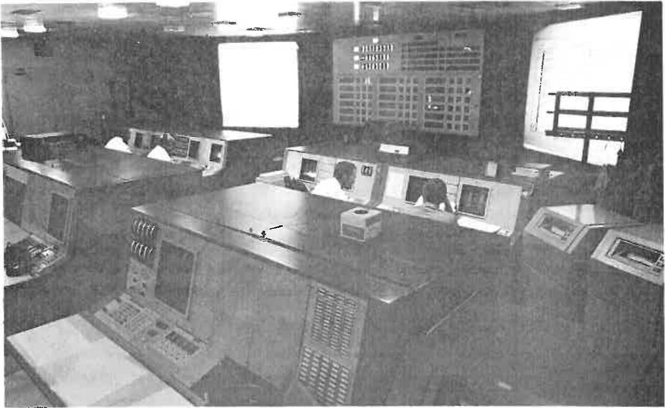
Station Control and Display Consoles
